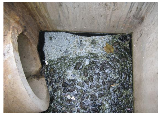
Example of floatables from an illicit discharge to a storm sewer.
