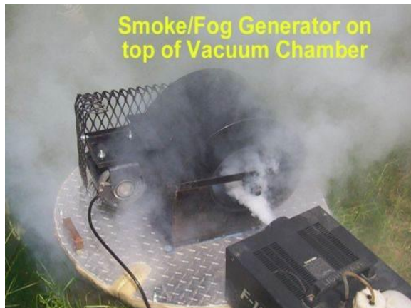
Example of smoke testing equipment injecting non-toxic smoke into a storm sewer.
