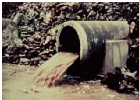
Illicit discharge example – Sediment laden runoff
