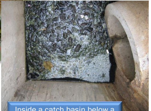
Inside a catch basin below a poorly maintained dumpster area located 50 ft from the recreational area of a lake.
