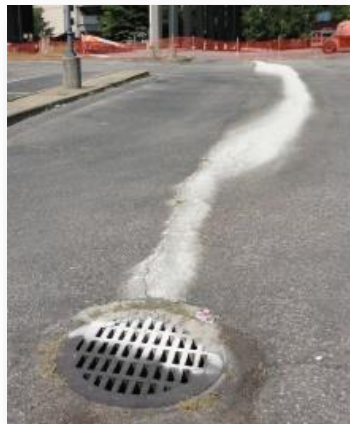
Indicator: Deposits from concrete washout
