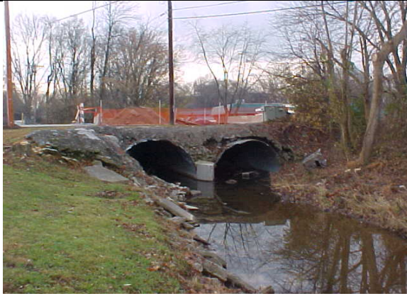
This bridge replacement includes stream isolation to minimize sediment discharge to the stream.
