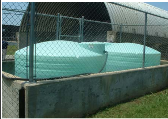
Secondary containment is used to protect the area in the event of a spill
