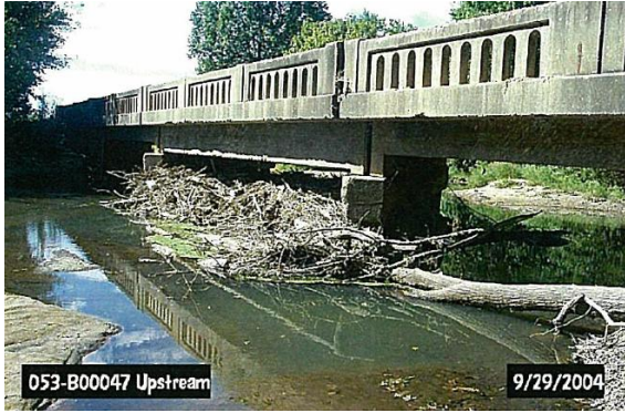
Large debris jam on bridge.
