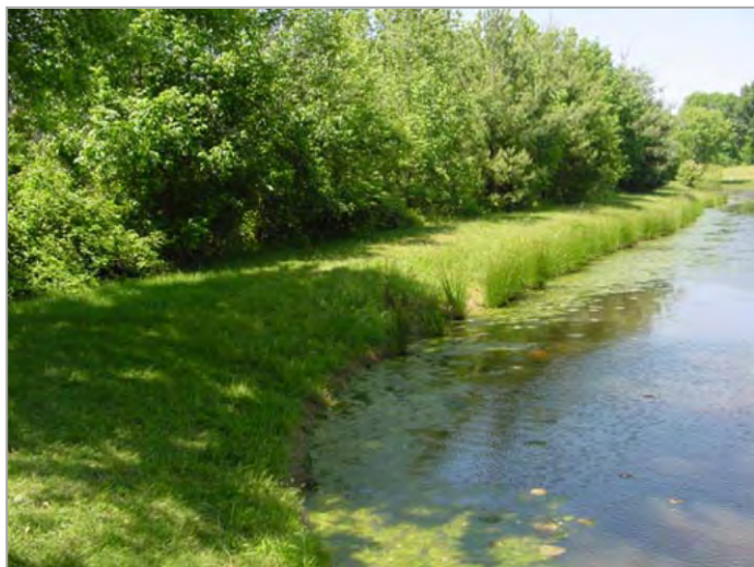
Figure 5: Excessive woody vegetation on dam embankment
