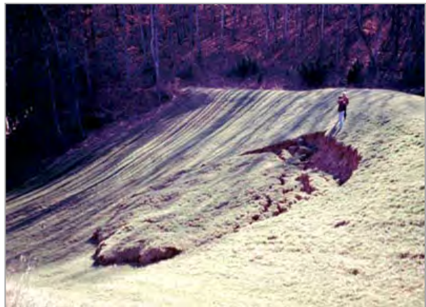
Figure 18: Soil slump failure of embankment
