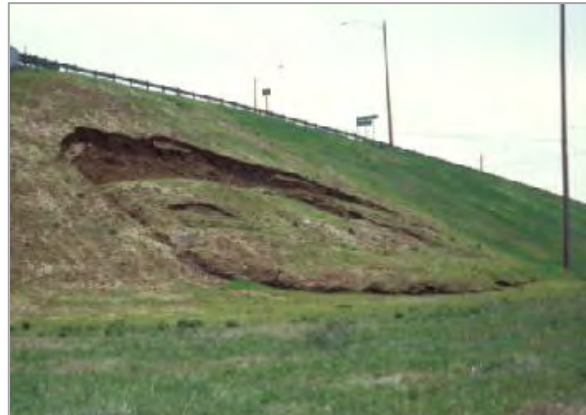
Figure 13: Example soil failure along embankment
