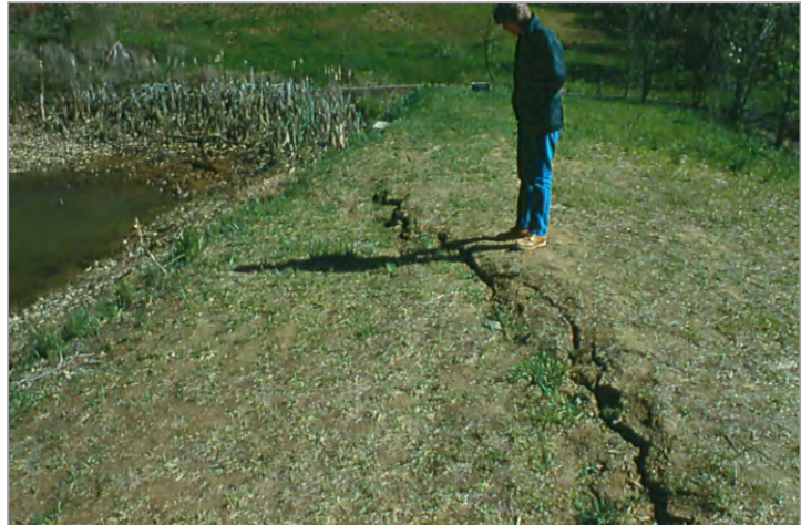
Figure 14: Longitudinal crack along top of embankment
