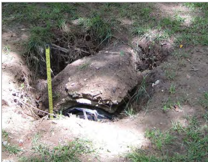
Figure 15: Voids on the surface from failing pipe joint
