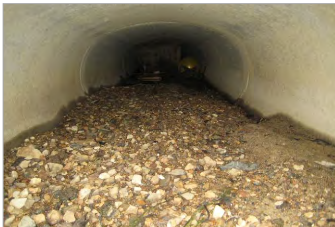
Figure 8: Sediment / debris accumulation in pipe
