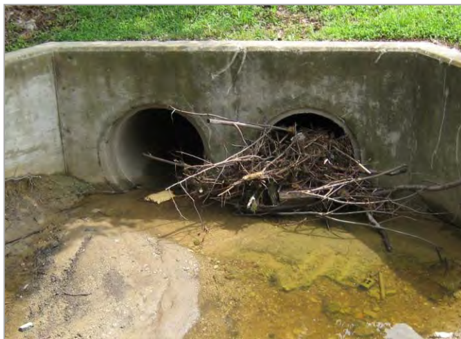
Figure 16: Blockage caused by inadequate maintenance
